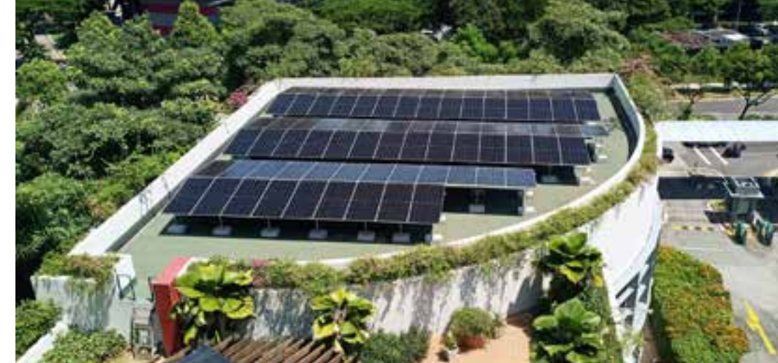
New photovoltaic cells, Asia Campus
